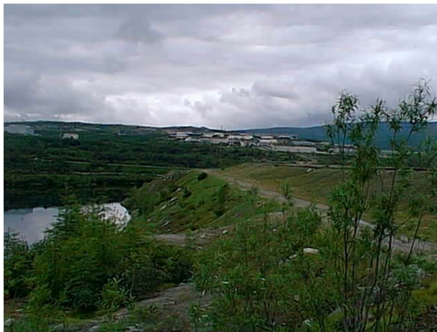
7 of 7 - View of downstream face of Magadan Power Plant coal ash dam showing the toe of the dam located in the floodplain of the Magadan River
