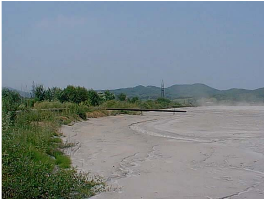
3 of 7 - View of crest of dam showing how full completely full it is with coal ash
