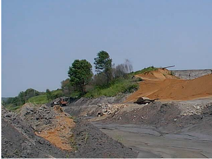
2 of 7 - View of drainage canal filled with fly ash and construction equipment removing portions of toe of dam
