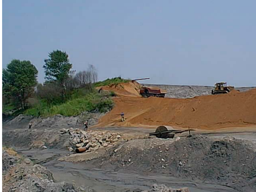
1 of 7 - View of the breach area being filled in also showing the height of the dam, the discharge point for emergency drainage pipe at the base of the breach area, the slope of dam and the height of mature trees growing in dam
