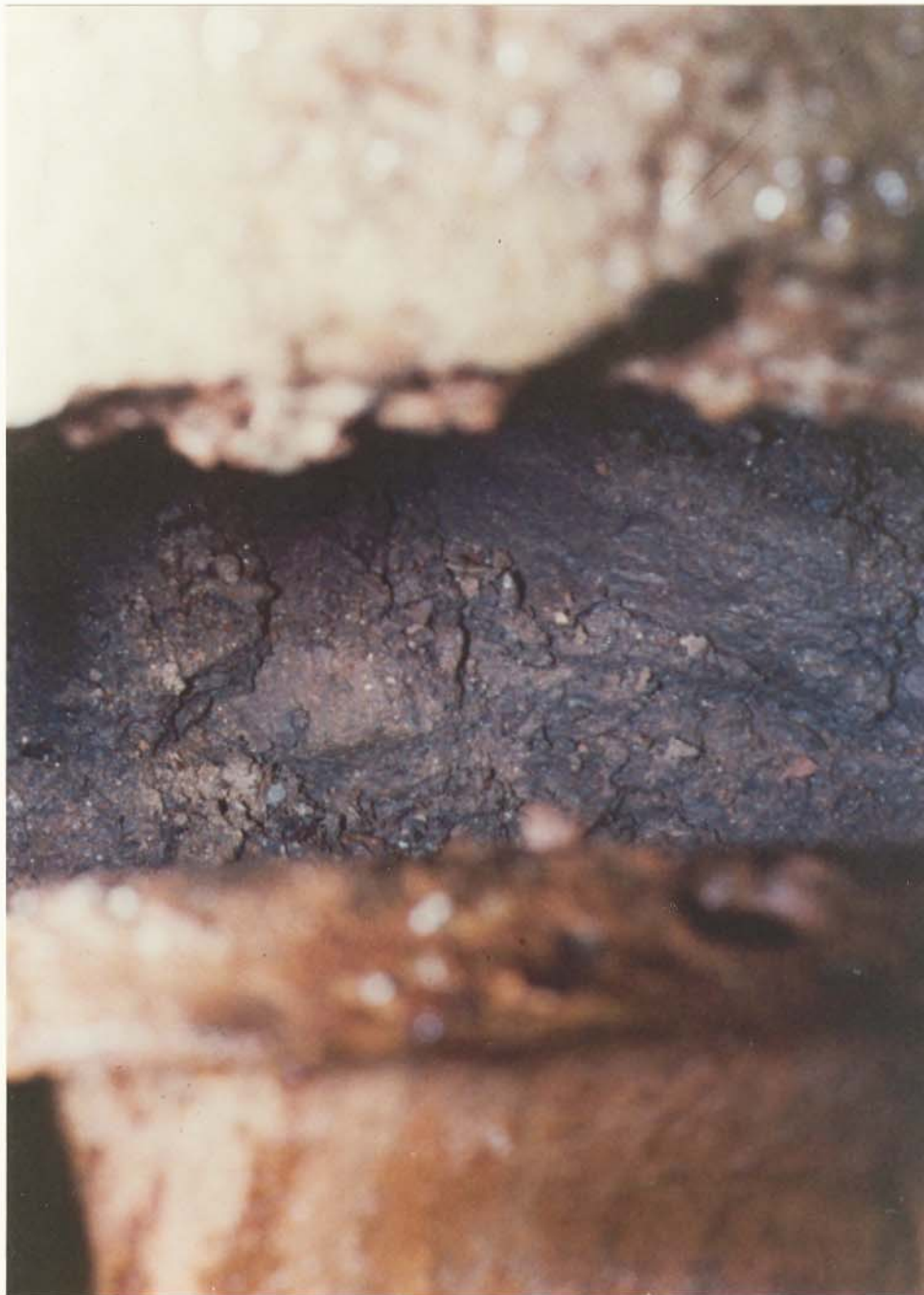
Plate 2. A closeup of the washout zone just below the Culebra Dolomite in the Waste Shaft.
