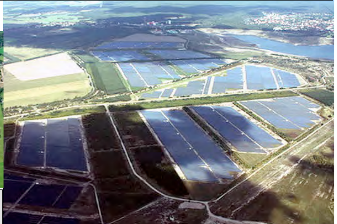
Senftenburg, Germany - 166 MW photovoltaic system being built at former open pit mine - 78 MW in operation in 2011 - at:
