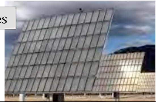
Questa, New Mexico Molybdenum Mine – 1.25 MW photovoltaic system – in operation on decommissioned portion of a tailings pile
